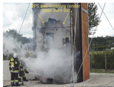
Figure 18. 67 min from the start - firefighters watering E_1 for safety reasons
