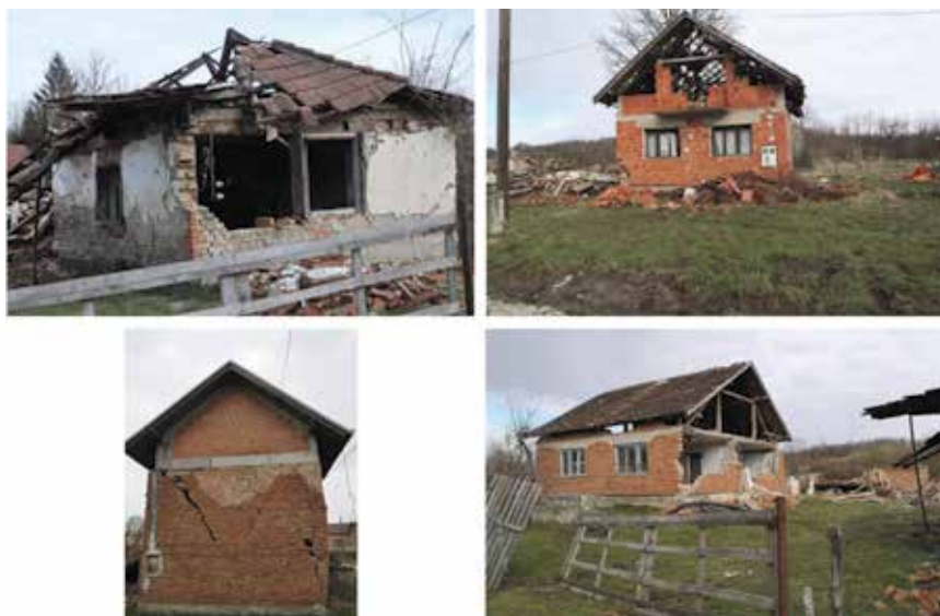
Figure 24. Photos of some severely damaged and demolished houses in Majske Poljane
