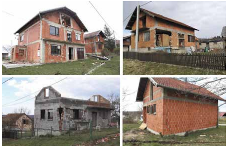
Figure 23. Characteristic damage to family houses in Novo Selo Glinsko
