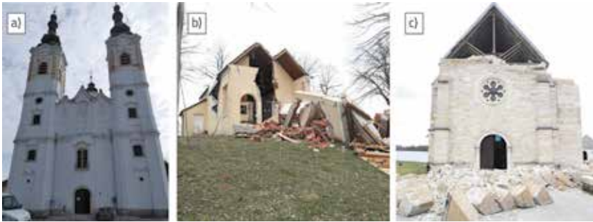
Figure 26. Some of the churches heavily damaged in the earthquake: a) St. Mary Magdalene Church in Sela; b) SS. Blaise and Benedict Church in Novo Selo Glinsko; c) Church of the Assumption of the Blessed Virgin Mary in Gora
