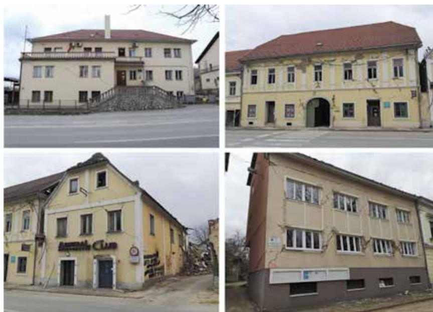
Figure 20. Buildings in Petrinja with typical damage to load-bearing façade walls
