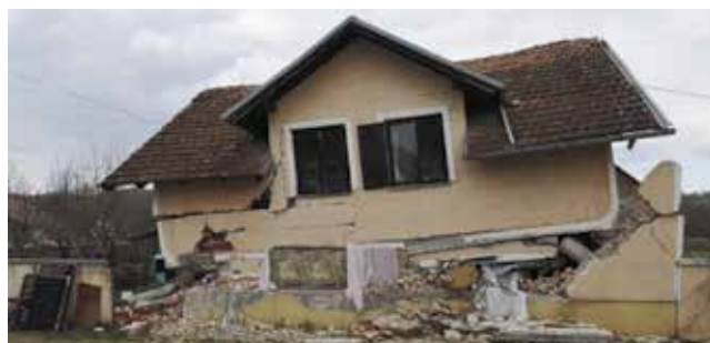
Figure 25. A family house in Prekopa was demolished due to flexible ground floor and force of the earthquake
