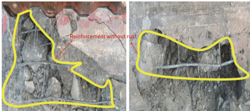
Figure 10. Corrosion of steel bars
