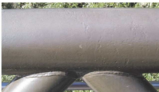
Figure 1. Hot finished circular hollow section with pitted surface [3]
